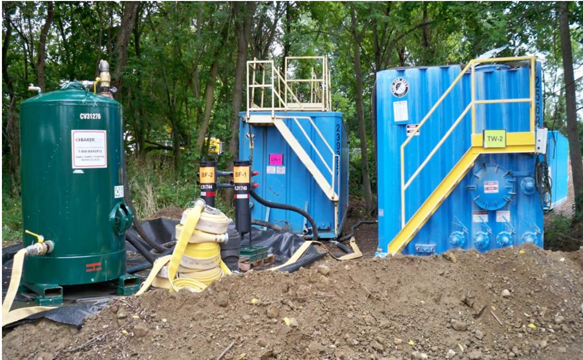
Photo #19: Water filtration system (under construction): Water storage tanks, bag filters (2) and carbon filter (1 of 2 shown)
