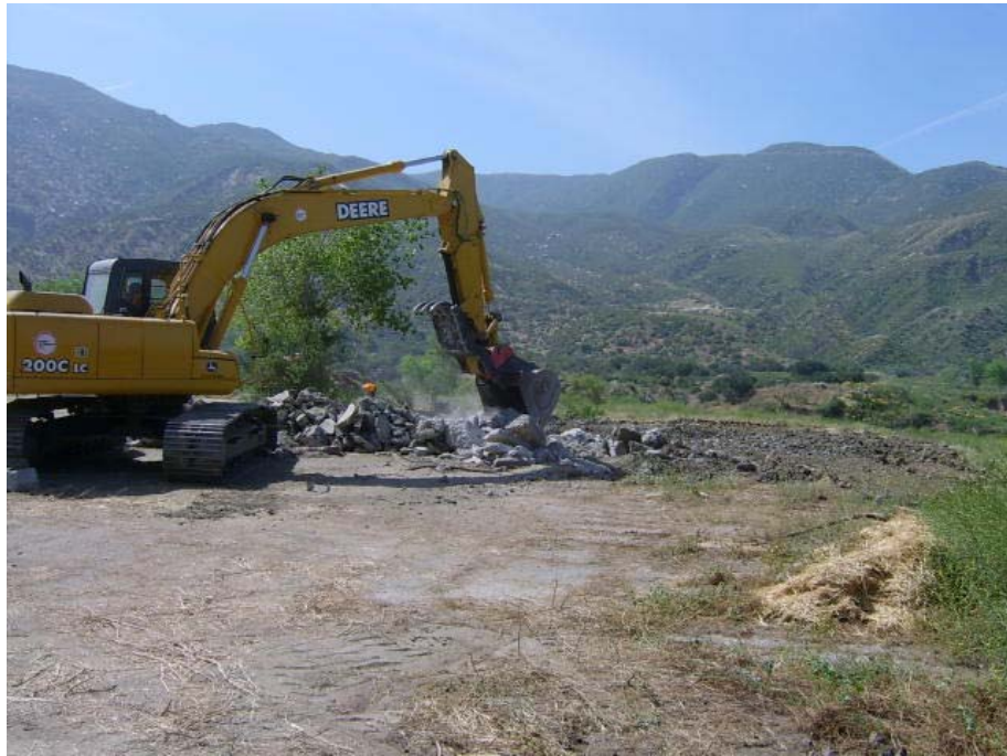
Photo 15: Offset Area 8 – Removal of former helicopter weapons test area pads (note flagging of burrows and use of small load displacement mats)
