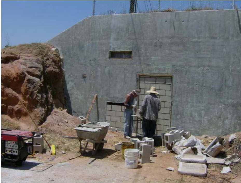
Photo 3: Exhibit H Item 6 – Remove access to Building 304 through placement of concrete block in previous door and duct openings
