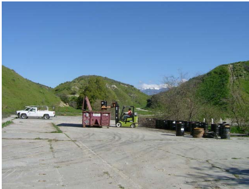
Photo 16: Site 2 - Removal of drums containing soil from drilling boring activities. Soil contained in drums was dumped into roll-off bins for disposal and empty drums were transported off-site for recycling
