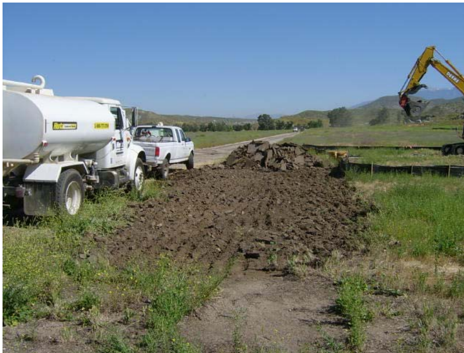
Photo 12: Offset Area 3 – Removal of former chemical storage building adjacent asphalt parking area
