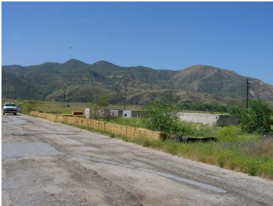
Photo 8: Offset Area 2 – Removal of former fuel slurry station (note silt fence and straw bales used to confine and exclude SKR while conducting trapping activities)
