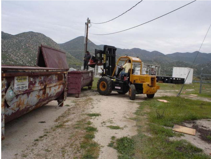
Photo 17: Site 1 - Removal of drums containing soil from drilling boring activities. Soil contained in drums was dumped into roll-off bins for disposal and empty drums were transported off-site for recycling.
