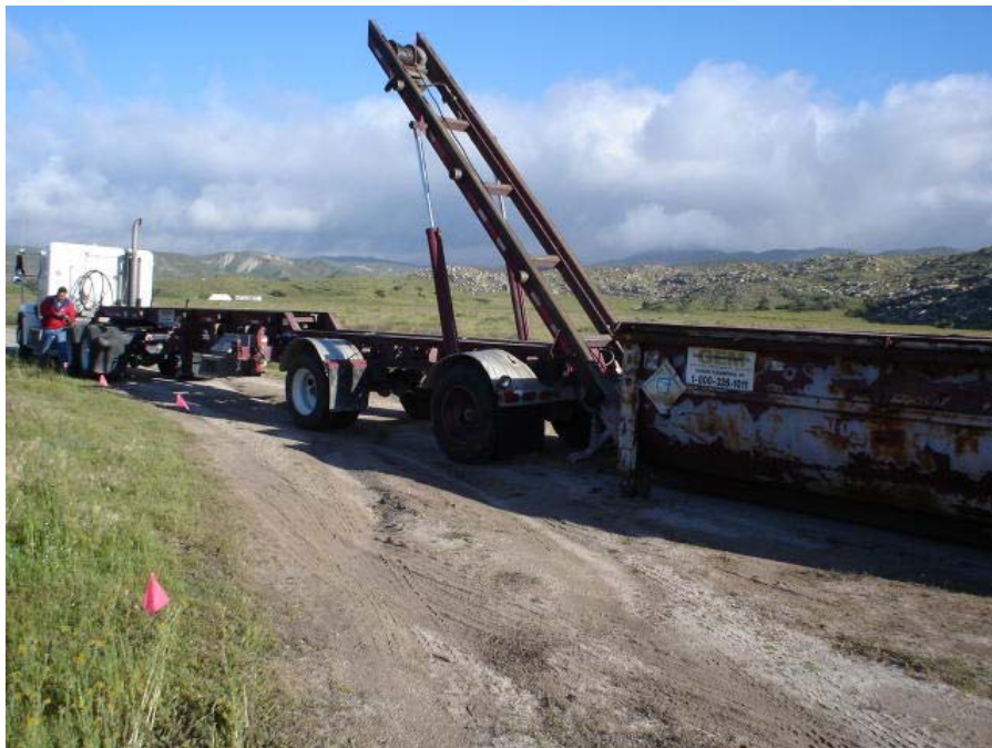
Photo 18: Site 1 - Removal of drums containing soil from drilling boring activities. Soil contained in drums was dumped into roll-off bins for disposal and empty drums were transported off-site for recycling. (Note use of pin flags to denote burrow locations)
