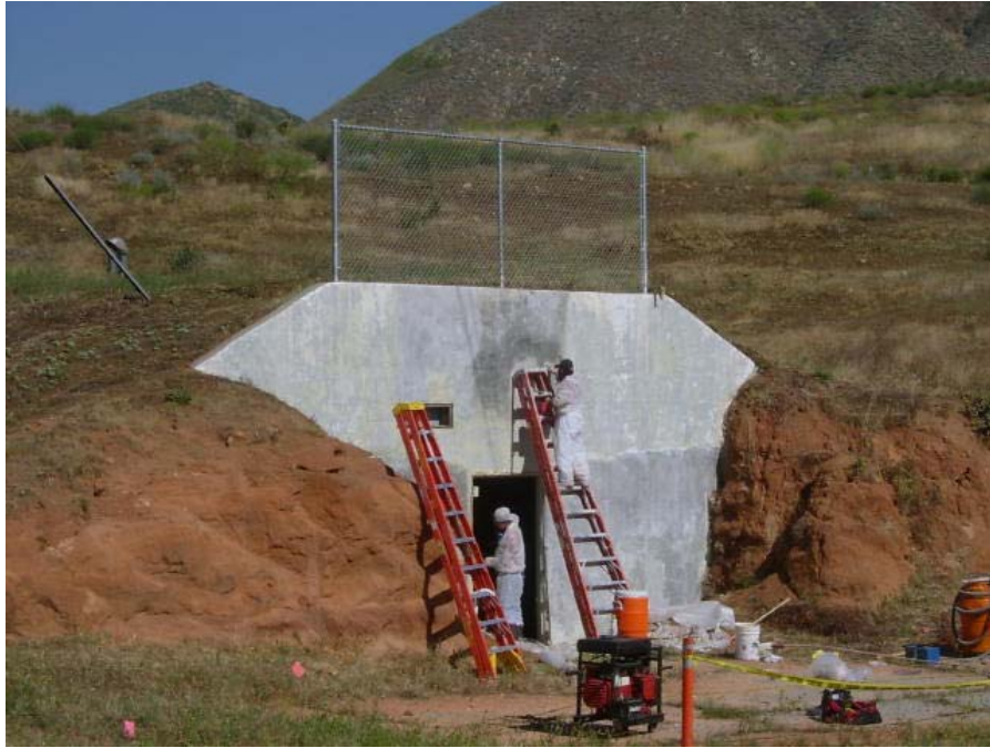
Photo 5: Exhibit H Item 10 – Re-abatement of Lead paint at Building 304 (abatement work at buildings 311, 312, and 325 similar)
