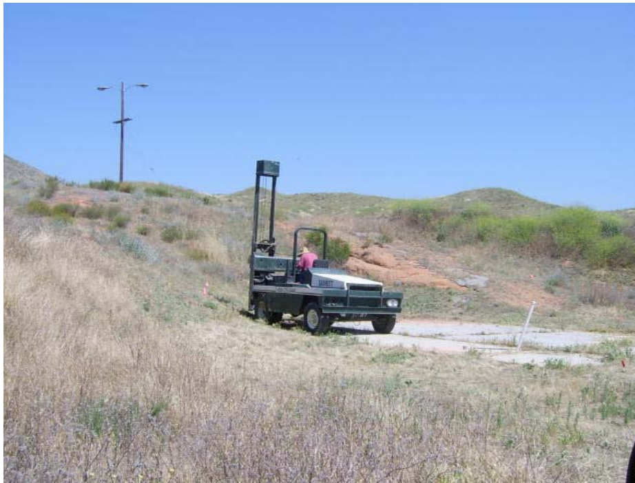
Photo 6: Use of stomper to fracture concrete prior to removal at all Offset Area locations
