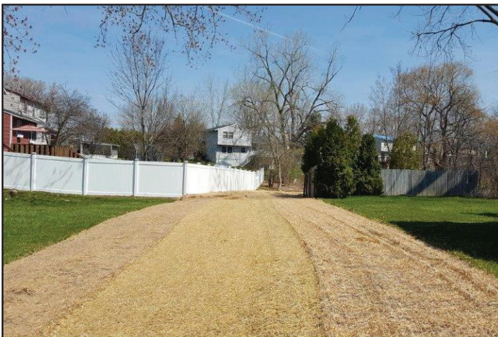
Brookview Lane access road restored with seed and covered with protective matting.
