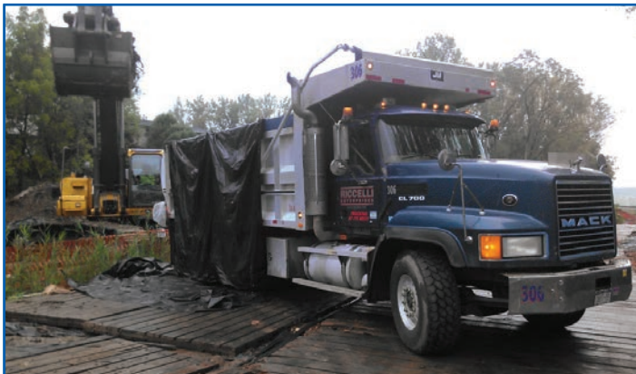
Loading soil from the site onto lined truck for disposal off site at a licensed landfill.
