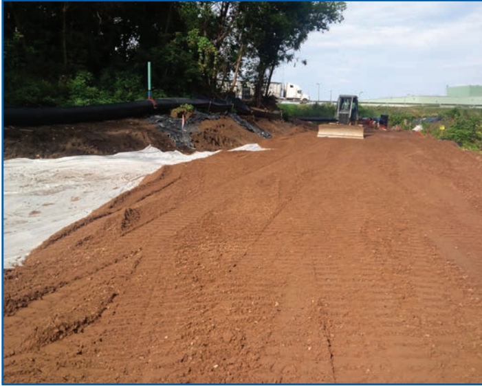
Backfill being graded in an upstream portion of the site that has been remediated.
