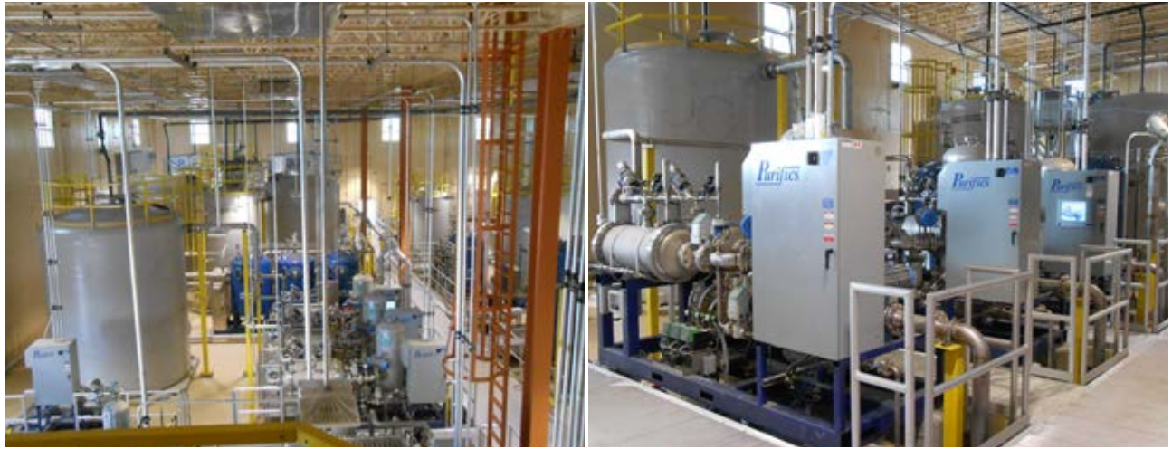
Images of the process equipment in the groundwater treatment plant.
