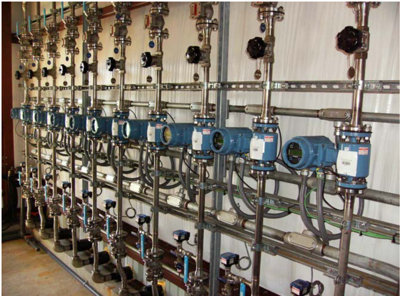
Extraction well manifold for interim groundwater treatment system.
